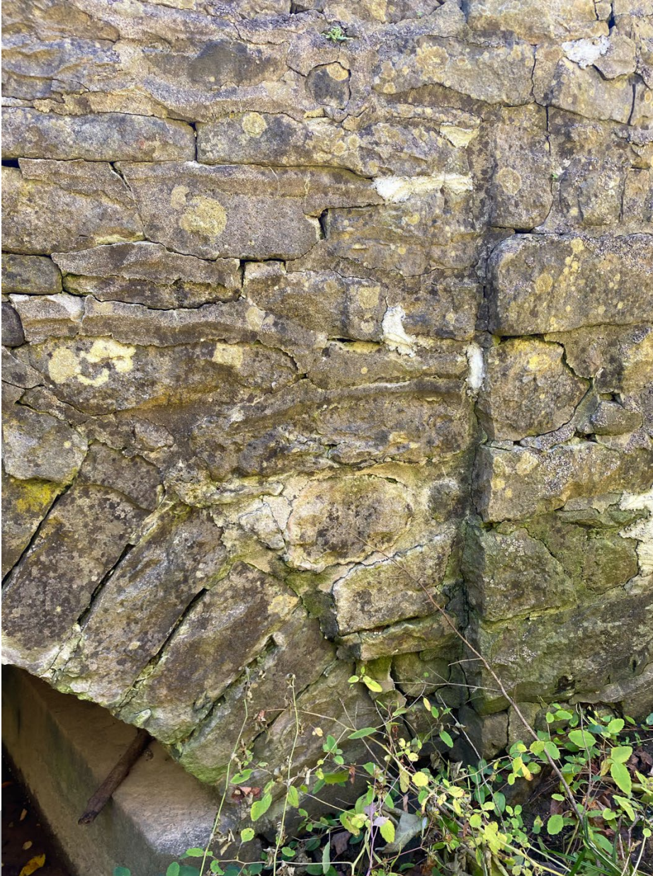
Photo 5: North (upstream) side of the bridge showing the vertical seam in the masonry.
