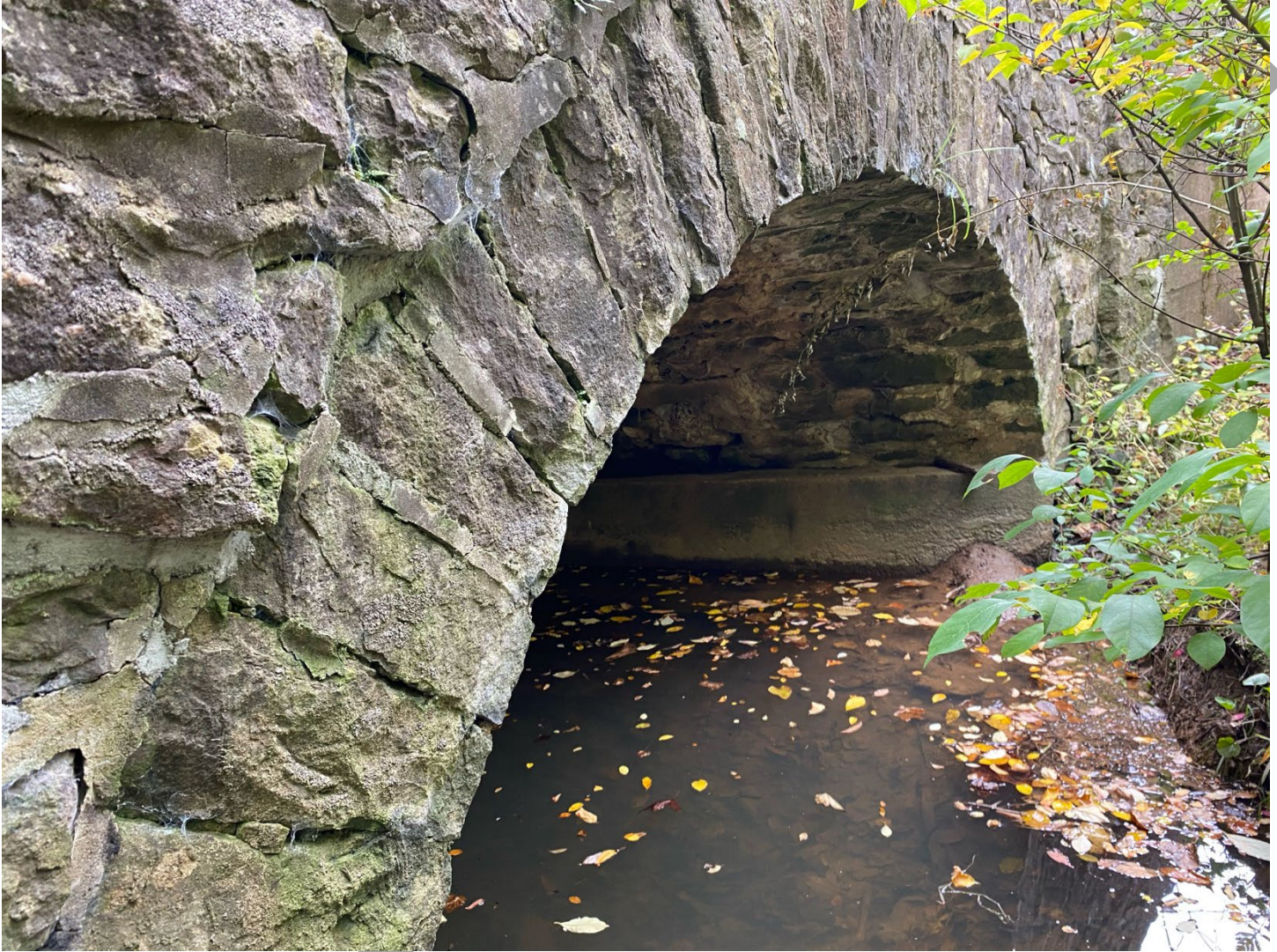
Photo 4: North (upstream) side of the bridge, view facing southwest showing the arch ring.
