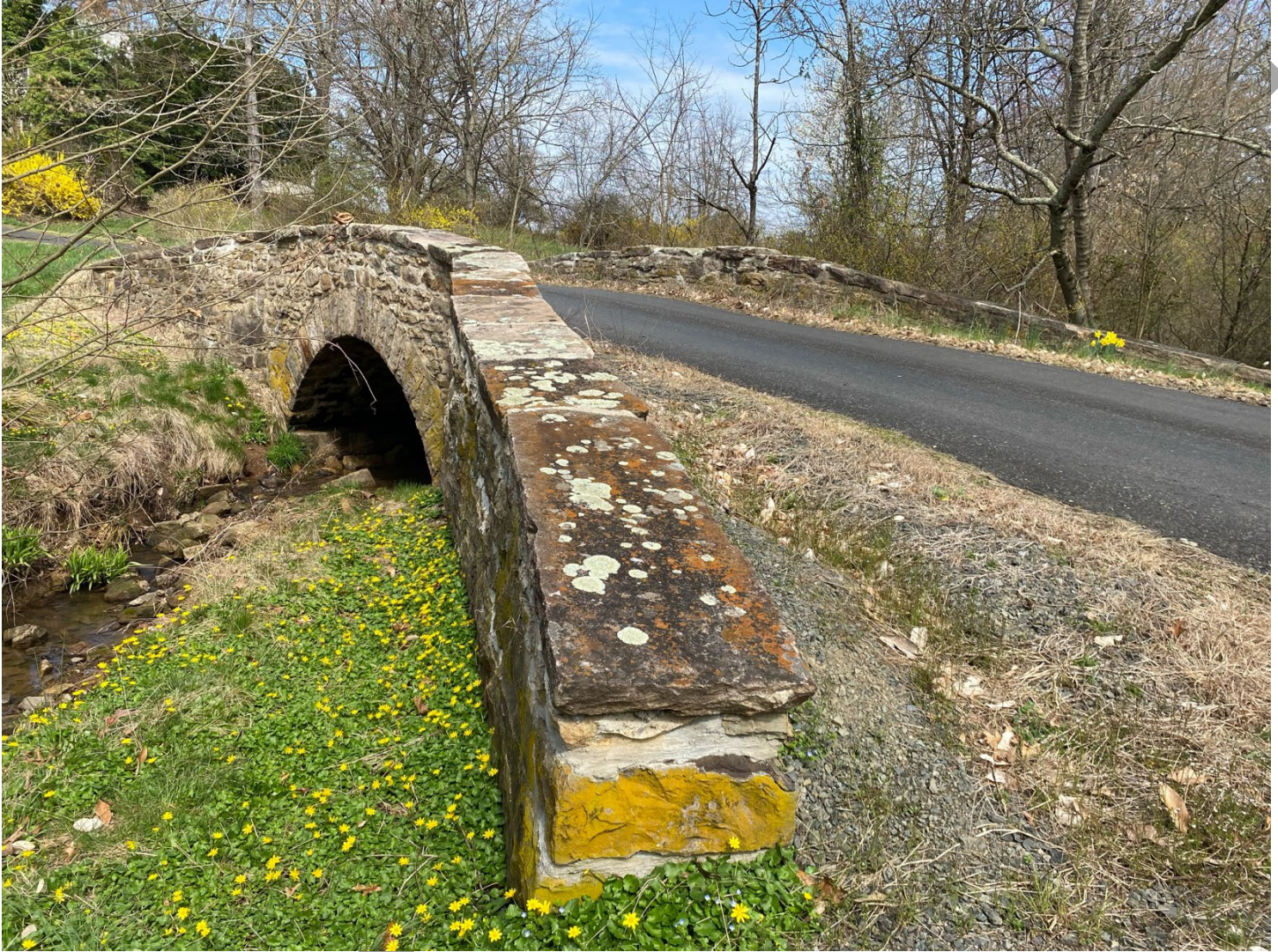
Photo 6. South (downstream) side of the bridge, view facing north west. Showing the original capstones.
