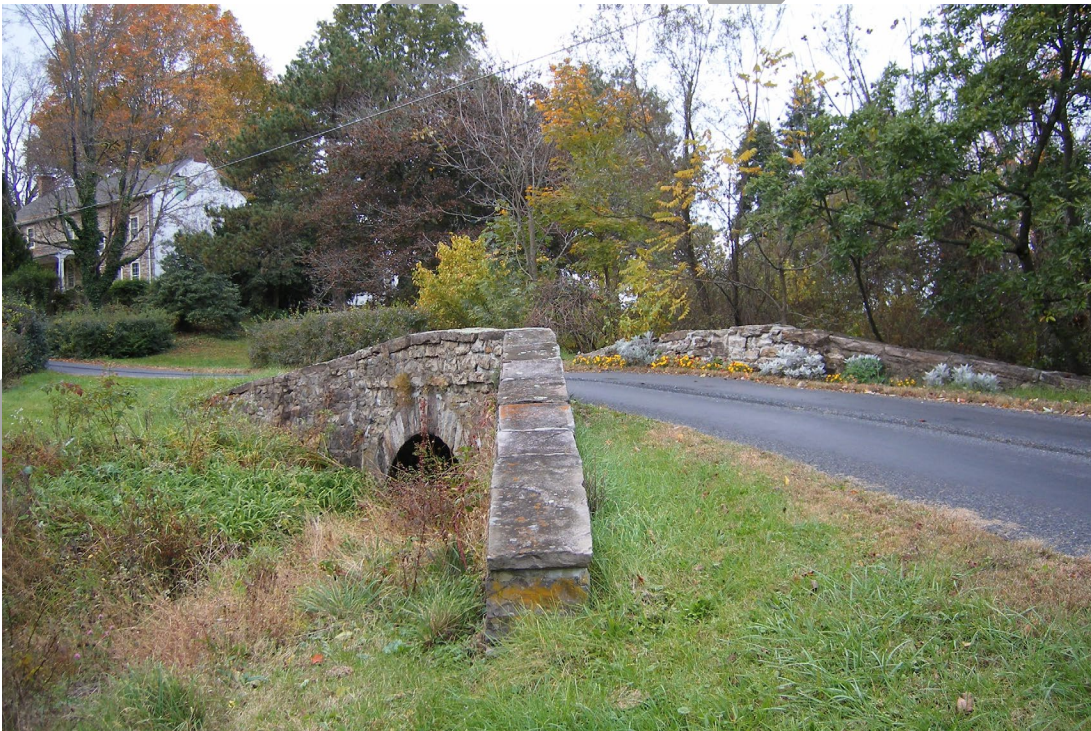
Illustration 10: 2008, Downstream side of the Yard Road stone arch bridge, view facing northwest. Showing the full inset panel prior to the reconstruction of the parapets. Complements of Marilyn Commings.
